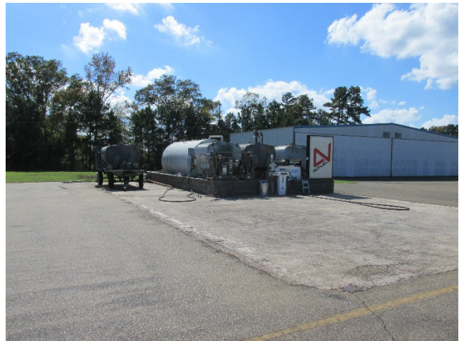
100LL Self-Service Fueling Facility
